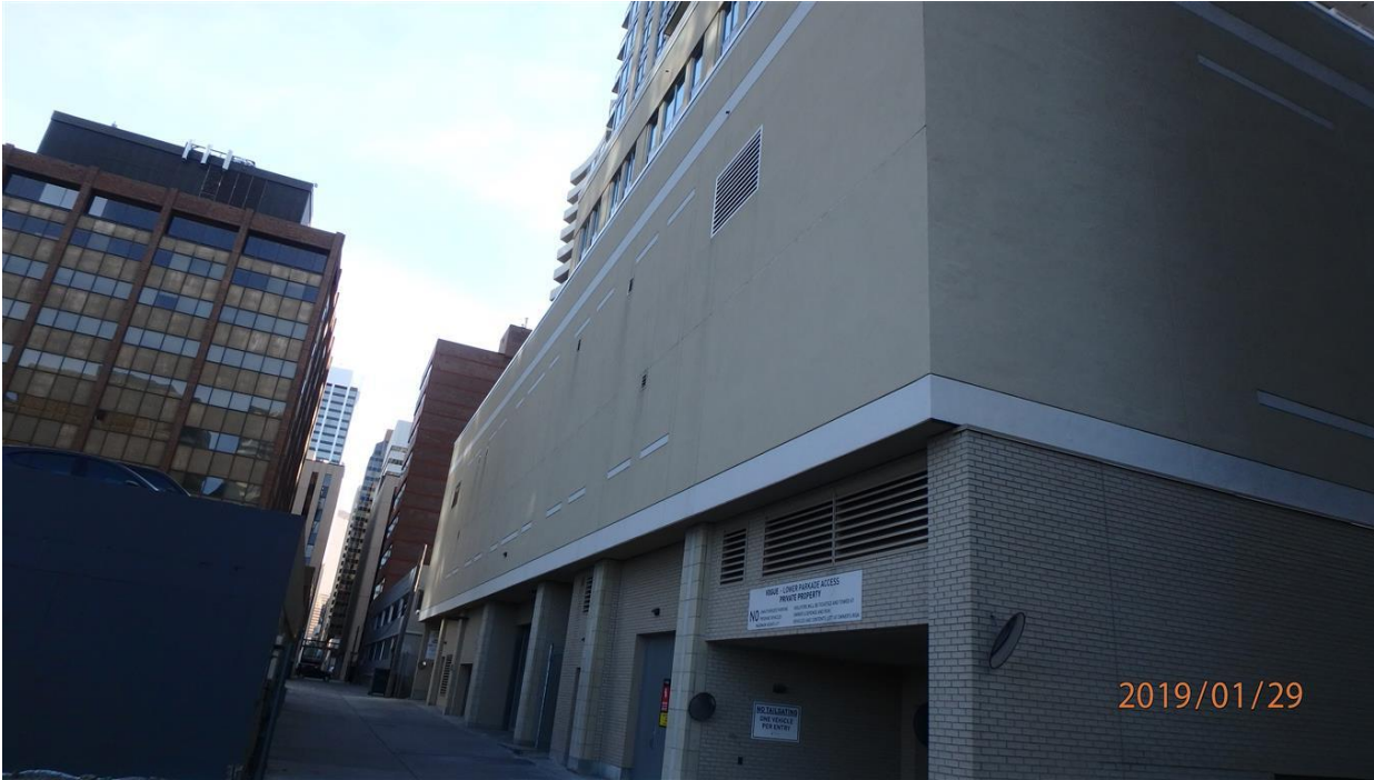
Photo 4 EIFS installed on building. Some water staining can be observed.
