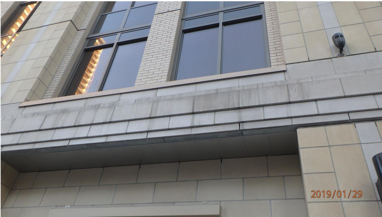
Photo 7 Water staining on stone masonry
