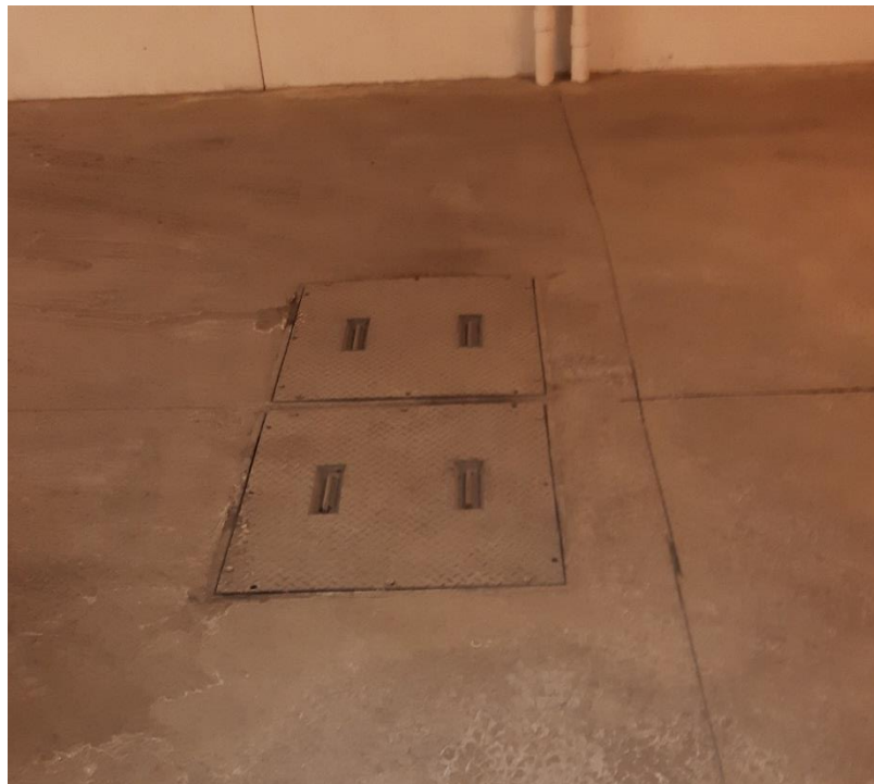
Photo 8 Sanitary sump floods during Fire Pump testing
