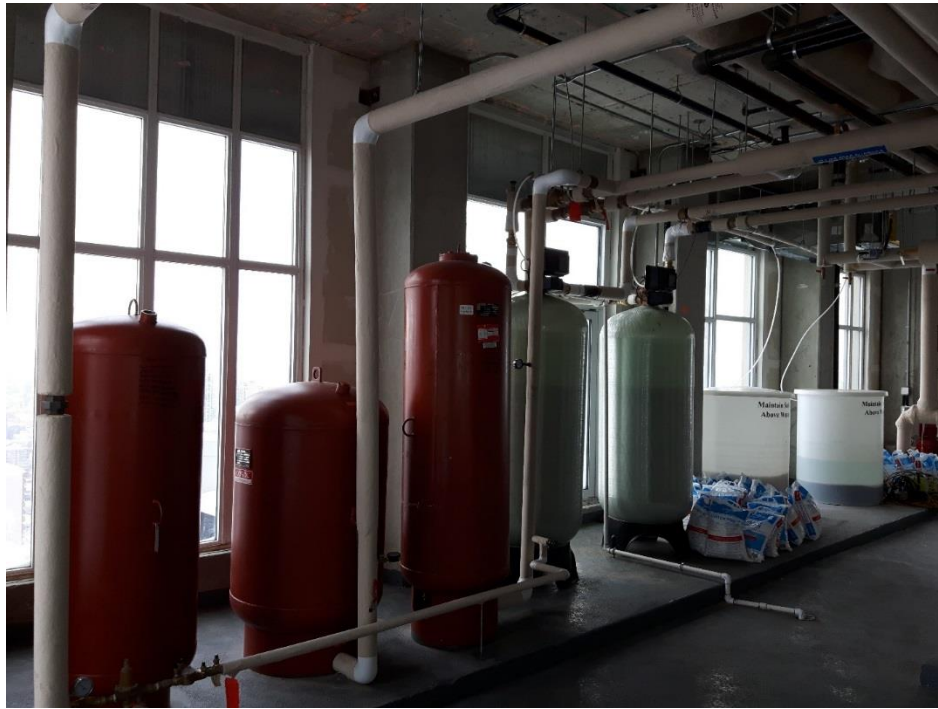
Photo 3 Water Softener System
