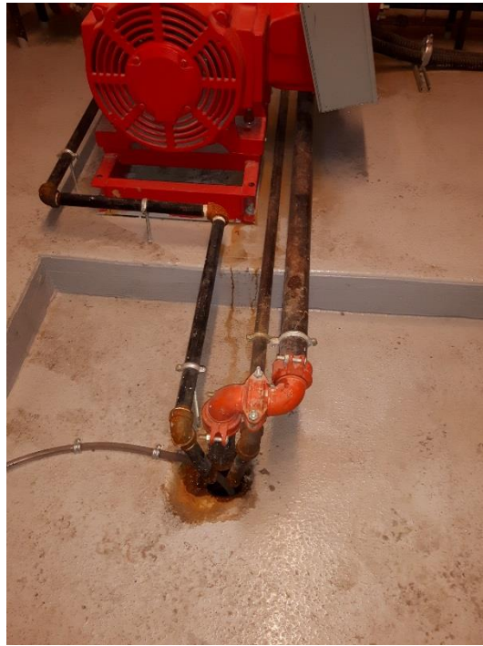
Photo 9 Fire Pump discharge down to sanitary sump in parkade
