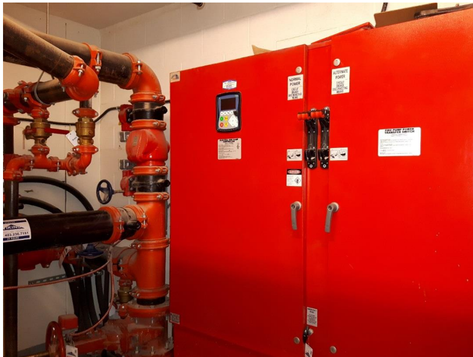
Photo 6 Fire Pump Controller
