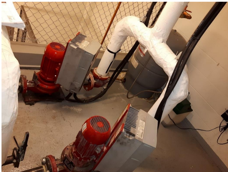
Photo 13 Glycol Circulating pumps
