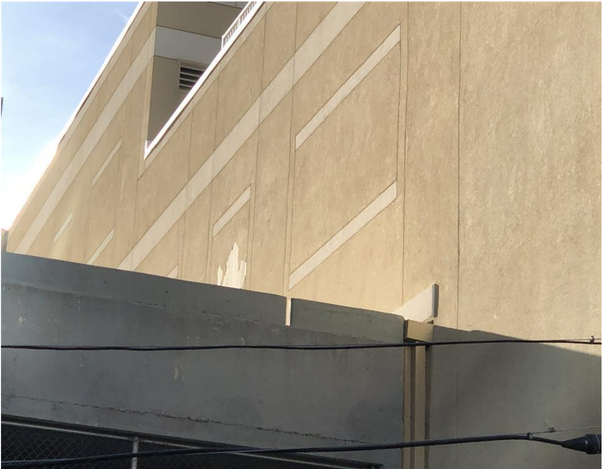
Photo 3 EIFS delaminating on East wall
