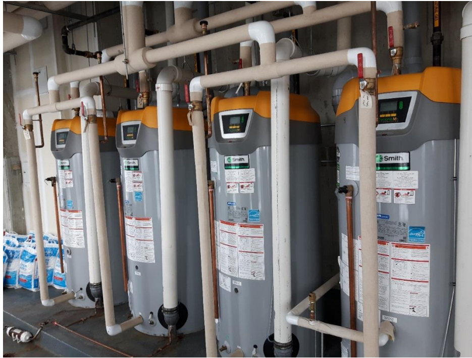
Photo 1 Domestic water heaters
