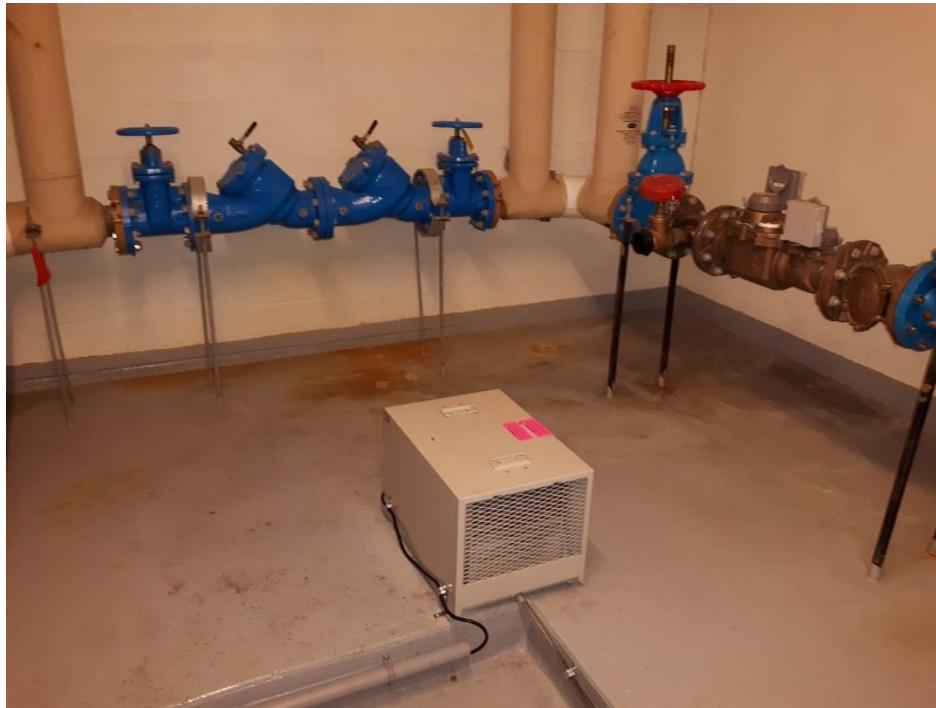
Photo 7 Dehumidifier unit in Water Entry room
