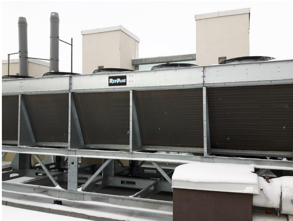
Photo 22 Dry Fluid Cooler
