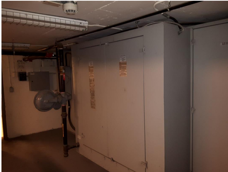
Photo 14 Parkade make-up air unit
