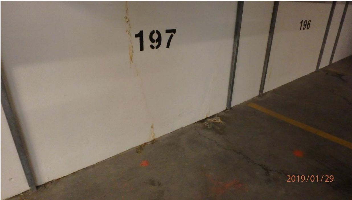
Photo 17 Leakage observed on concrete walls from interior of building
