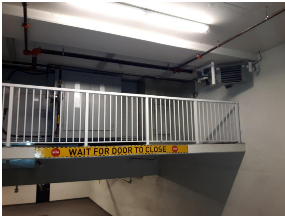
Photo 19 Parkade Make-up Air unit
