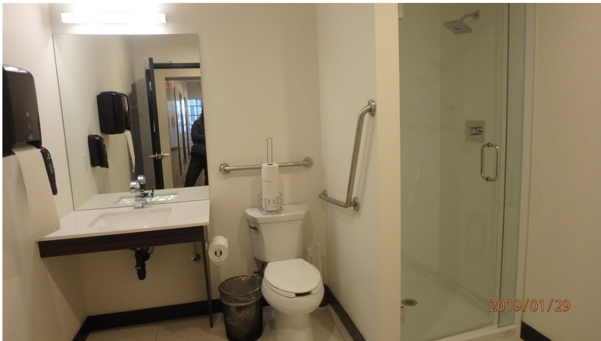
Photo 22 Amenities level bathroom
