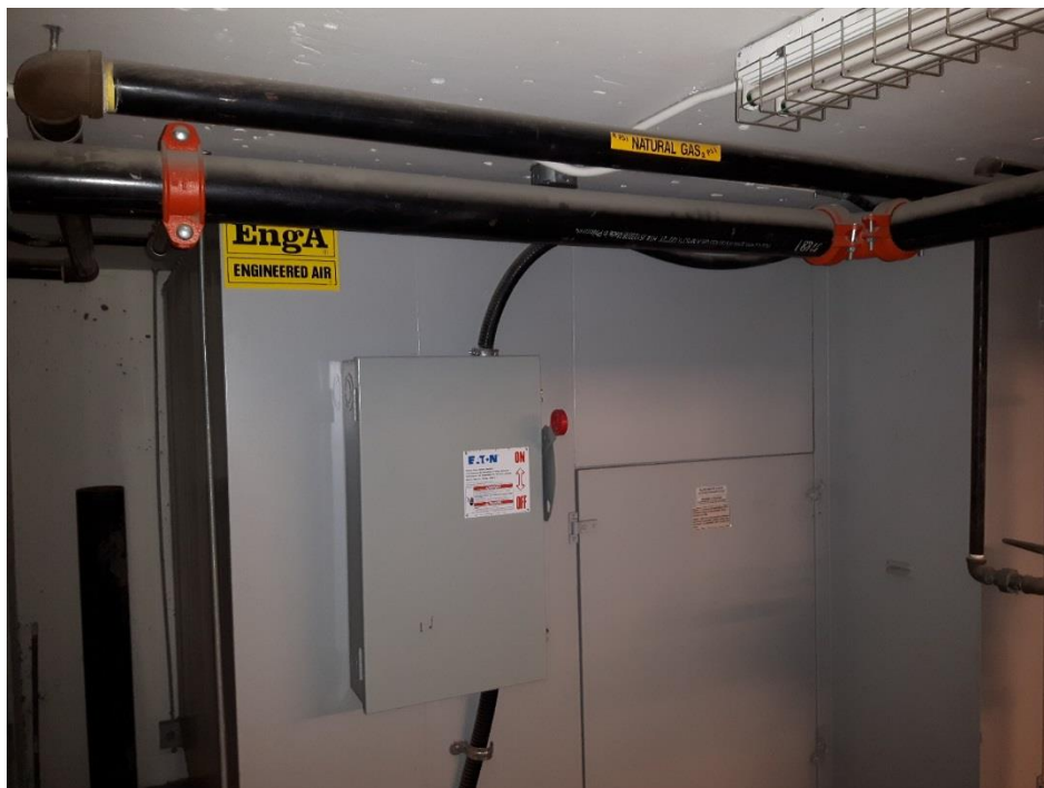
Photo 15 Parkade Make-up air unit
