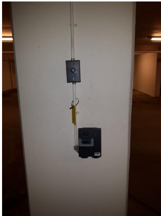
Photo 17 CO sensors in parkade
